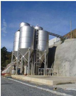
Waste water treatment facilities
